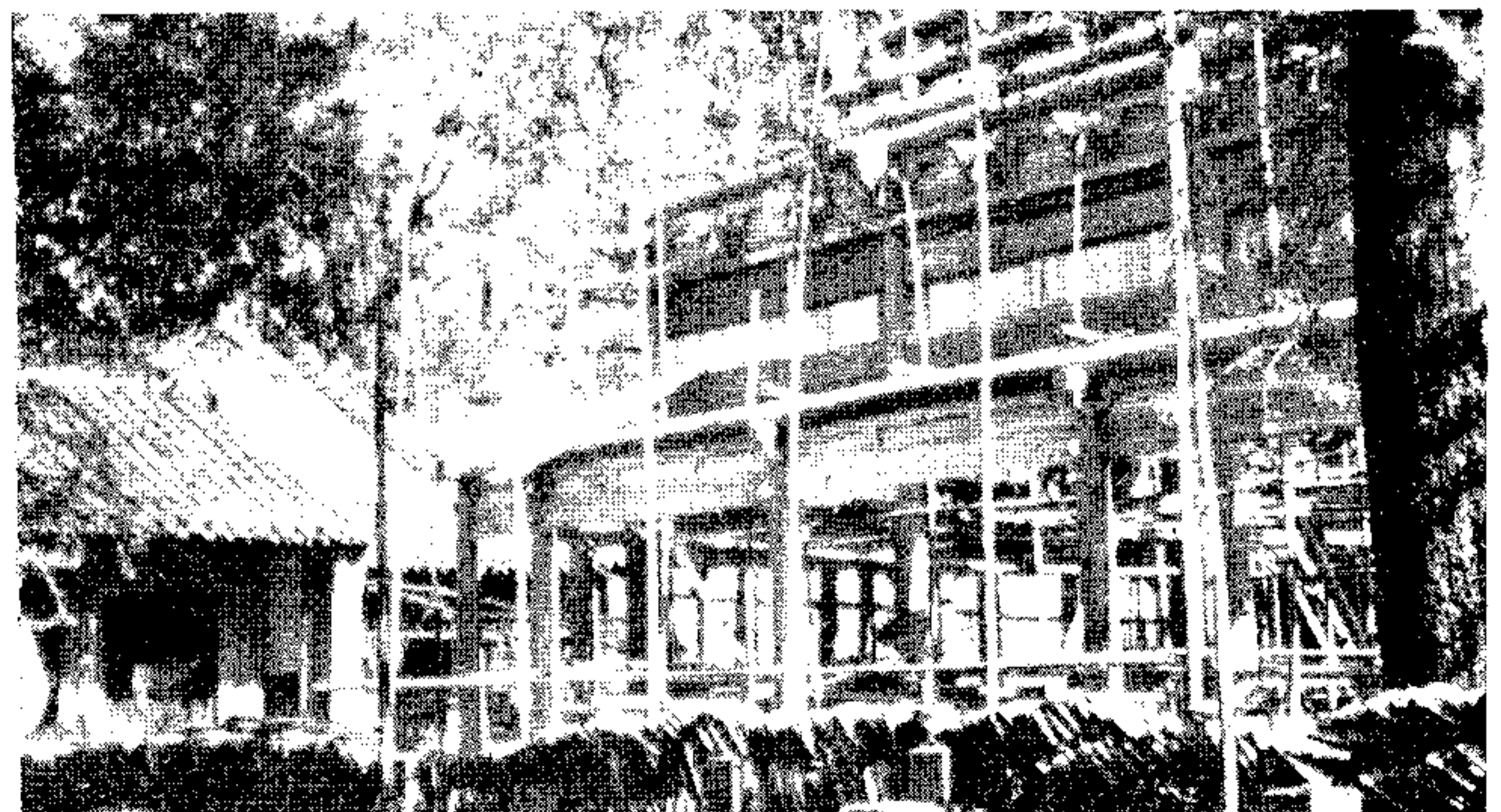
Jiao Shan : Tien Wang Dian, new temple under construction almost directly in front of Ding Hwei Si.
